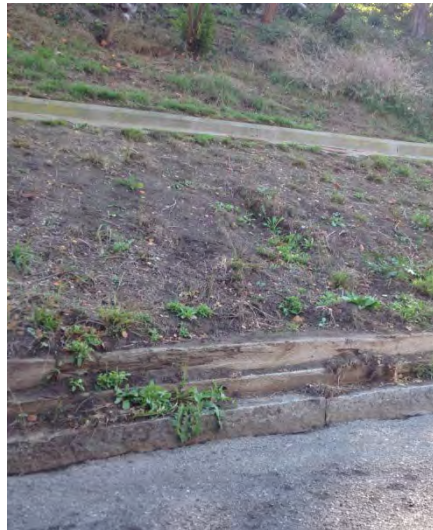
ERODED SLOPE, BUTTRESSED BY TEMPORARY RETAINING LOGS
